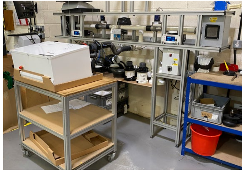
All MVHR are tested for air leakage
