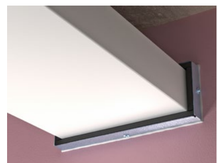
QRS Fire Sleeve installed in plasterboard partition
